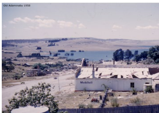
This rare photo shows the demolition of the Mobil Service Station & Garage at Old Adaminaby in 1958 prior to the lake flooding. (Photo source supplied by Justin Richardson of Adaminaby Ampol)
